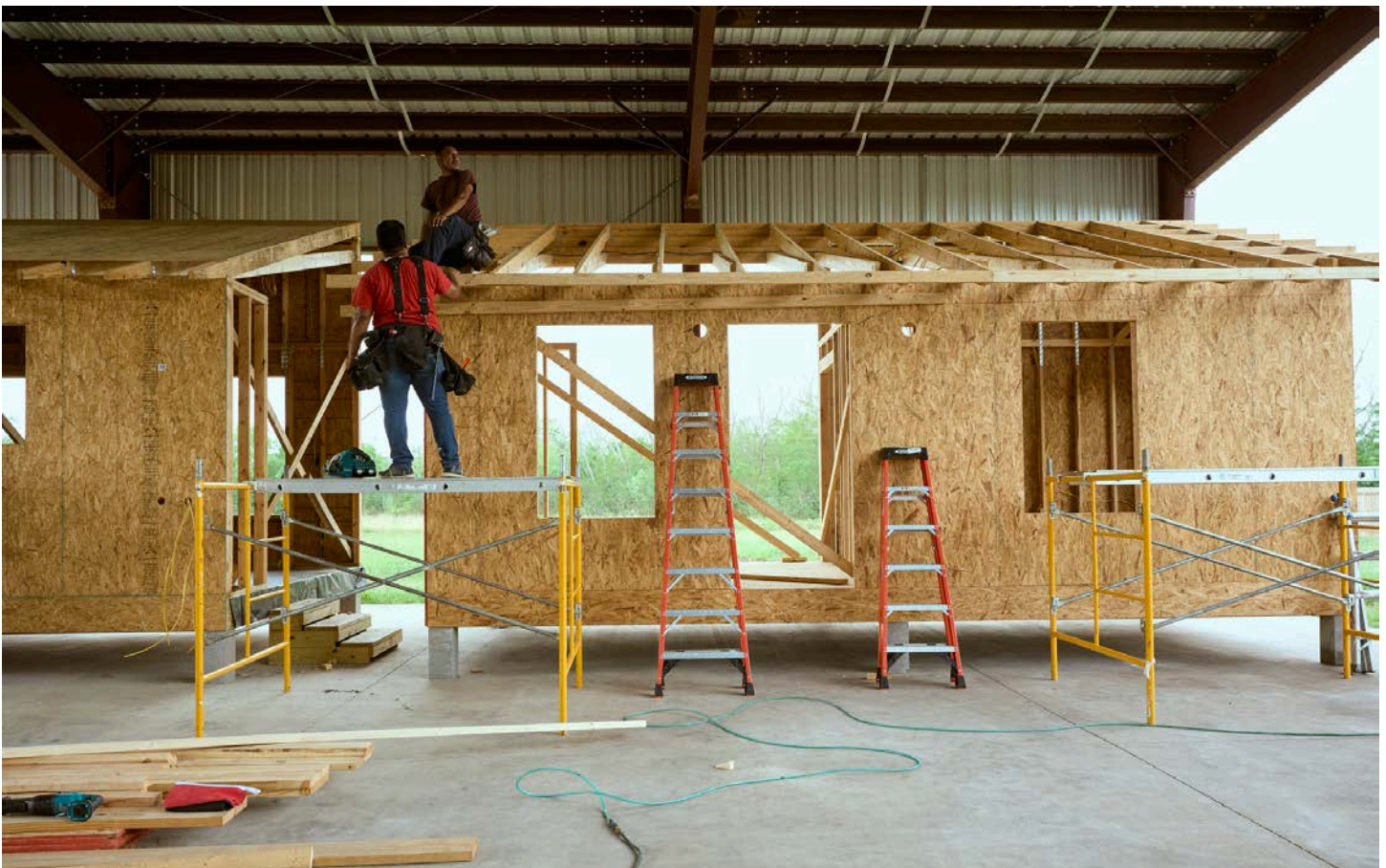
DreamBuild homes under construction at The Farm, an off-site manufacturing facility, in Los Fresnos, Texas.
