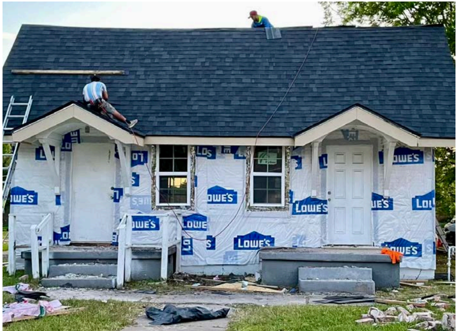
The Kendall Whittier Neighborhood Trust, a MINT in Tulsa, Oklahoma, renovates a duplex.
