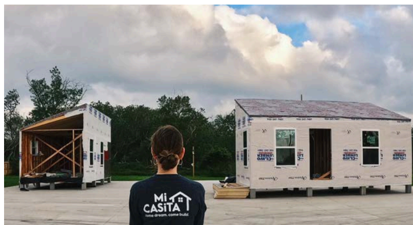
DreamBuild boxes, components of its "grow home" volumetric housing model, under construction in the Rio Grande Valley, Texas.
