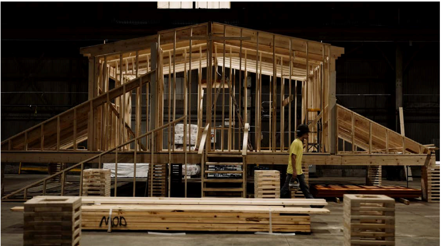
A Module home under construction at the Last Mile Facility in Carnegie, Pennsylvania
