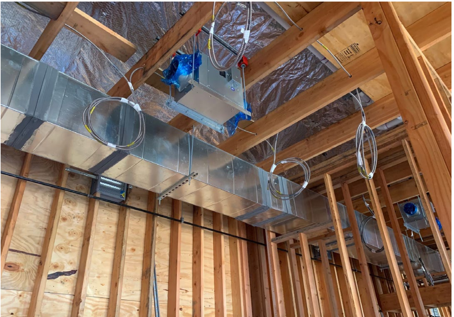
HVAC ductwork at Inwood Gardens
